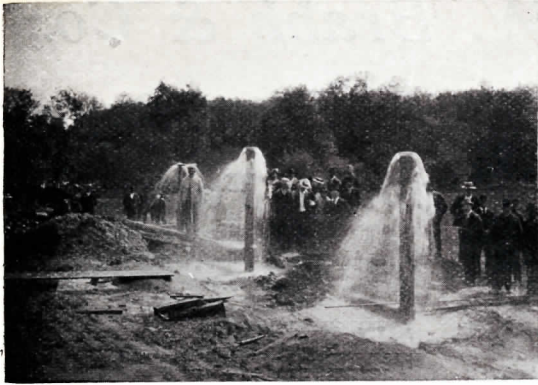
WATER WORKS WELLS.
